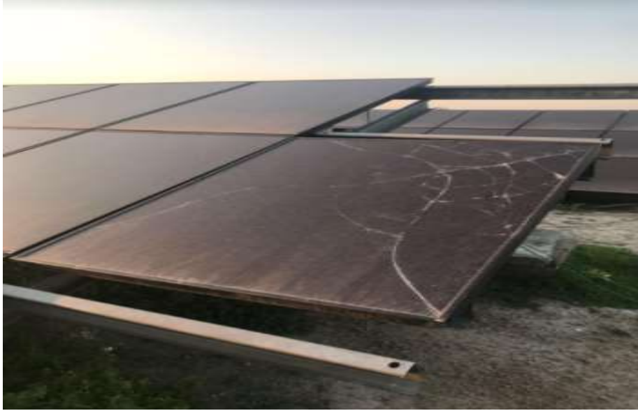
Figure 7: A sample of crack appear in PV array
