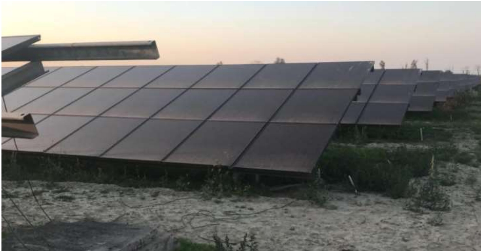
Figure 5: A sample of soiling appear in PV array
